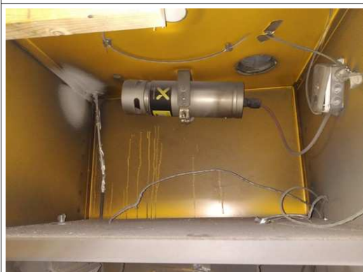
Ceiling of the ONOS Charge Safe after test
