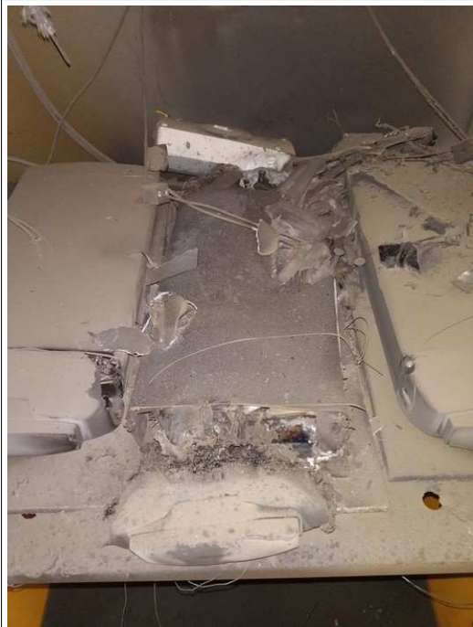
Battery after thermal runaway
