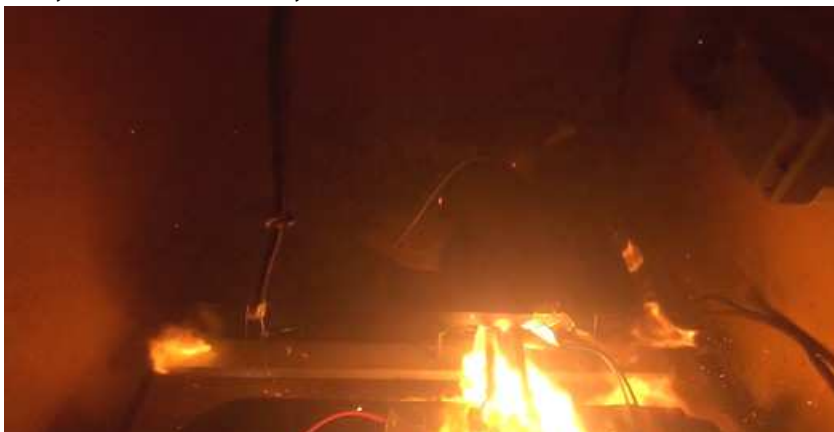
f4.1 Battery comes in thermal runaway
