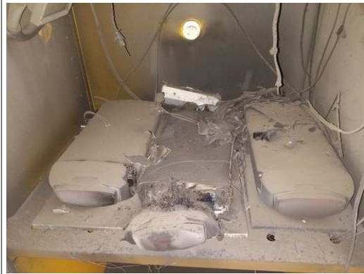
Batteries after the test
