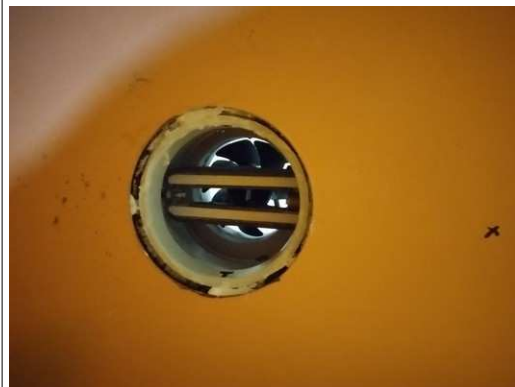
Fire damper and ventilator seen from inside
