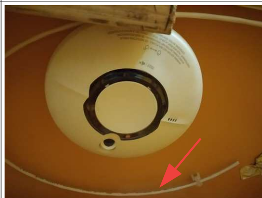
Smoke detector with around it the linear heat detection (red arrow)
