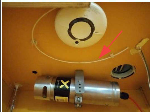
Ceiling ONOS Charge Safe with smoke detector and AF-X Fireblocker with linear heat detection (red arrow)
