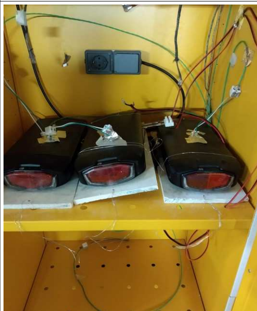
Batteries in ONOS Charge Safe
